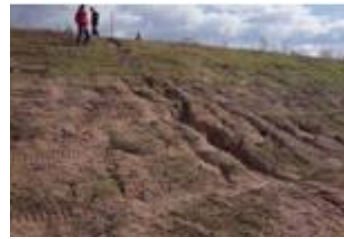
(2)堤防のり面の侵食
