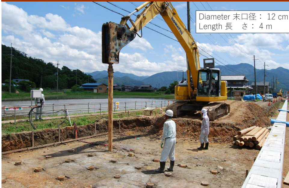
Soft ground improvement for road body (2011/7/8, Obama City) 道路路体の軟弱地盤対策 (2011/7/8, 小浜市)
