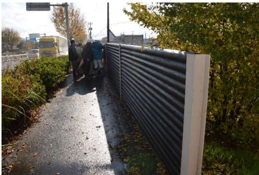
Sound Insulation Wall (Geba, Fukui City) 遮音壁 (福井市下馬)
