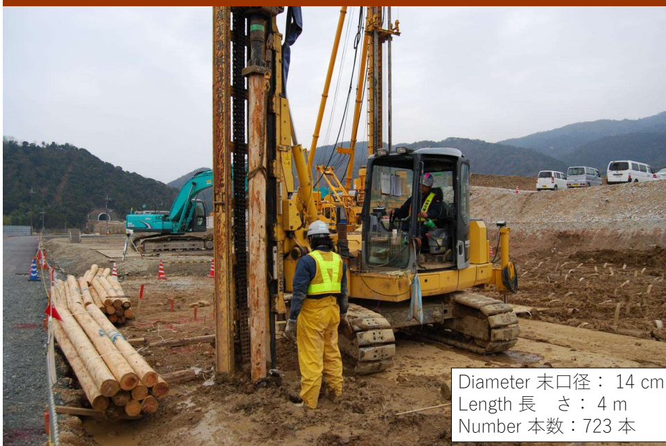
Soft ground improvement for embankment (2012/4/13, Mikata PA on Wakasa-Maizuru Expressway) 盛土の軟弱地盤対策 (2012/4/13, 若狭舞鶴自動車道三方PA)
